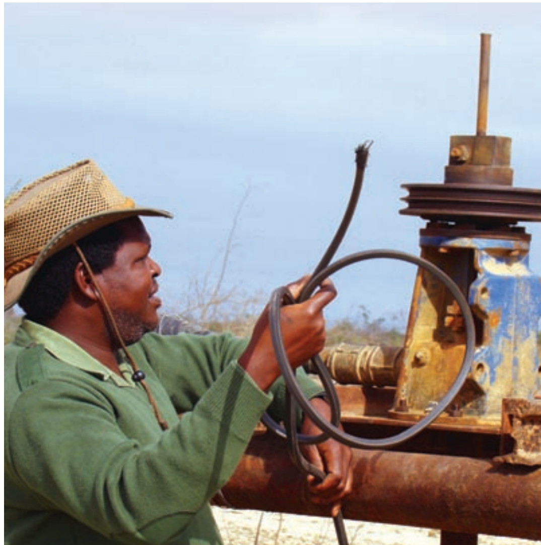
Repairs to water installations is a major activity that requires a dedicated water-maintenance team.
