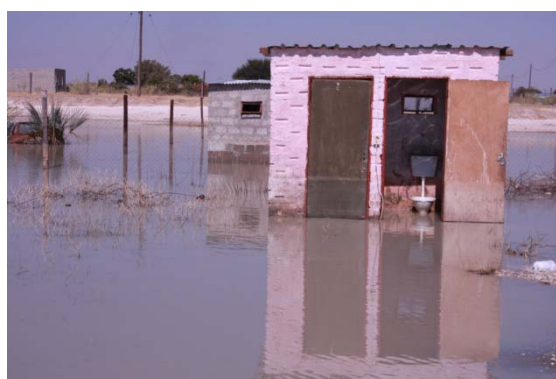
Figure 16: Flooded sanitation facilities
