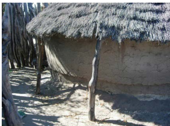
Figure 26: Houses damaged by flooding
